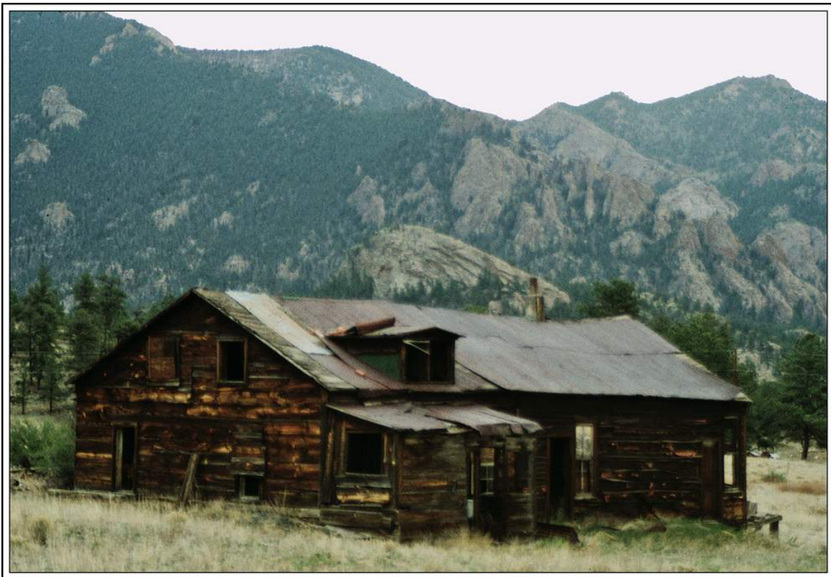
Abandoned building at Tarryall – This building may have been a store and possibly the post office. Photograph by William H. Bauer May 17, 2004
