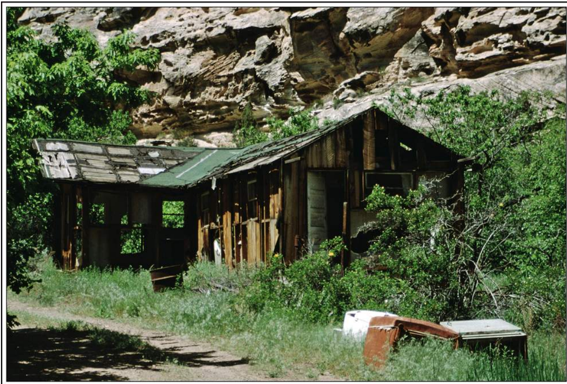
One of the abandoned buildings at the site of Cashin, Colorado Photograph by William H. Bauer May 22, 2003
